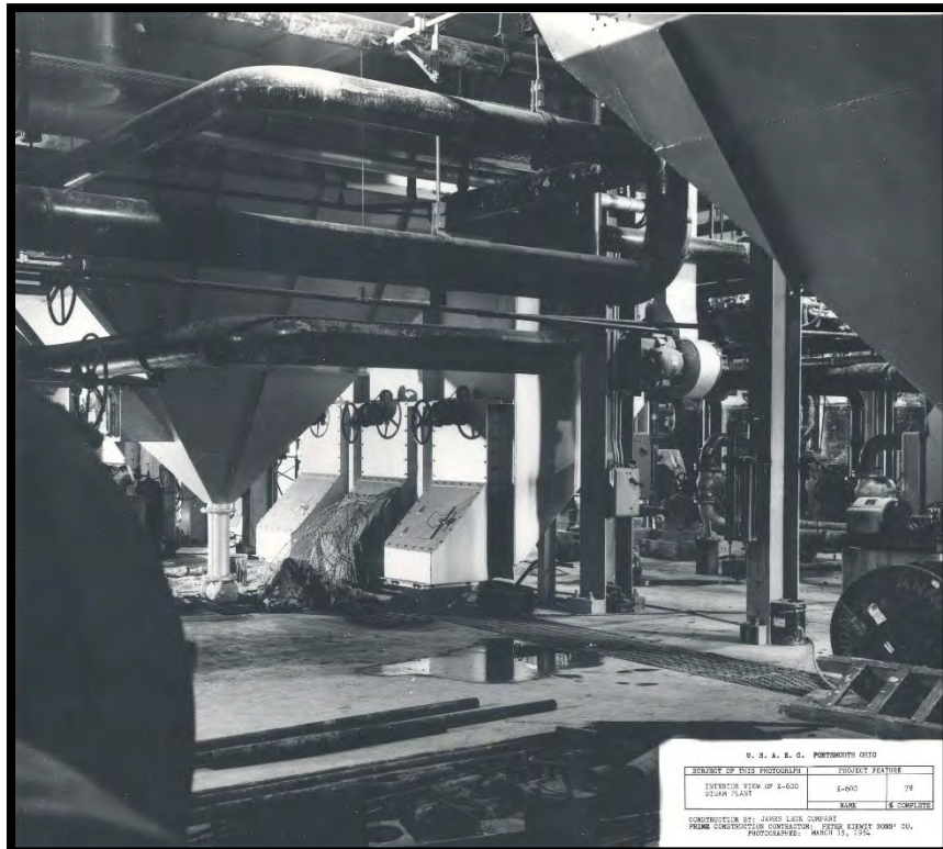
Figure 17: Interior View of the X-600 Steam Plant, March 1954
